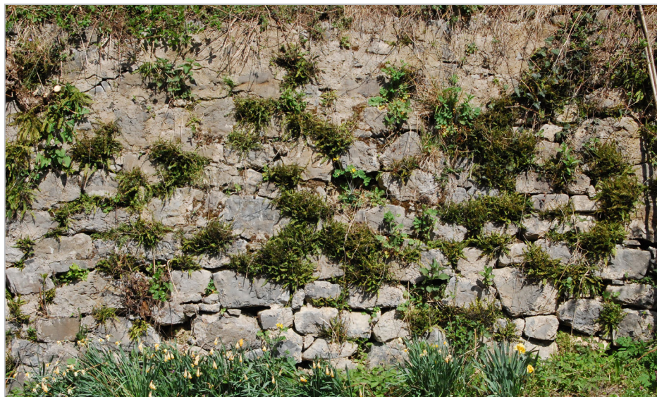
Fig. 9: Jurklošter, the retaining wall north of the monastery complex (Photo: M. Oter Gorenčič)
